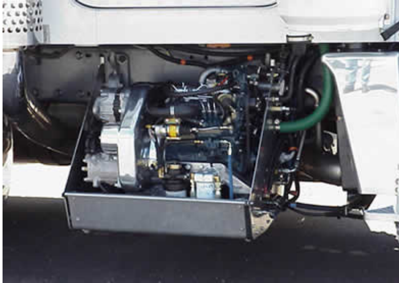
Figure 2.5.1. The picture above shows an internal combustion powered APU.
